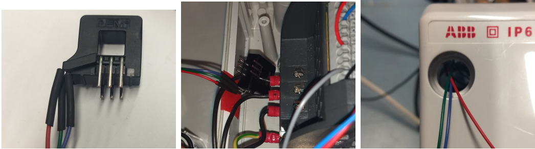
(a) Heat shrink on CT connections (b) CT mounted inside motor control box (c) Wires connected safely to CT
